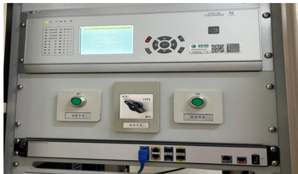
Figure 11 Second-level load control terminal for electric power
