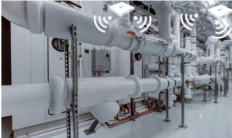
Figure 16 Underground pipeline monitoring
